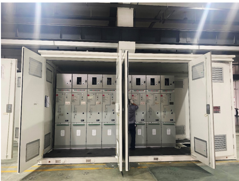
Secondary collector station
