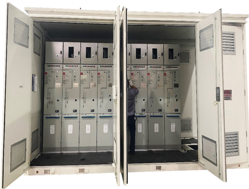
Secondary collector station
