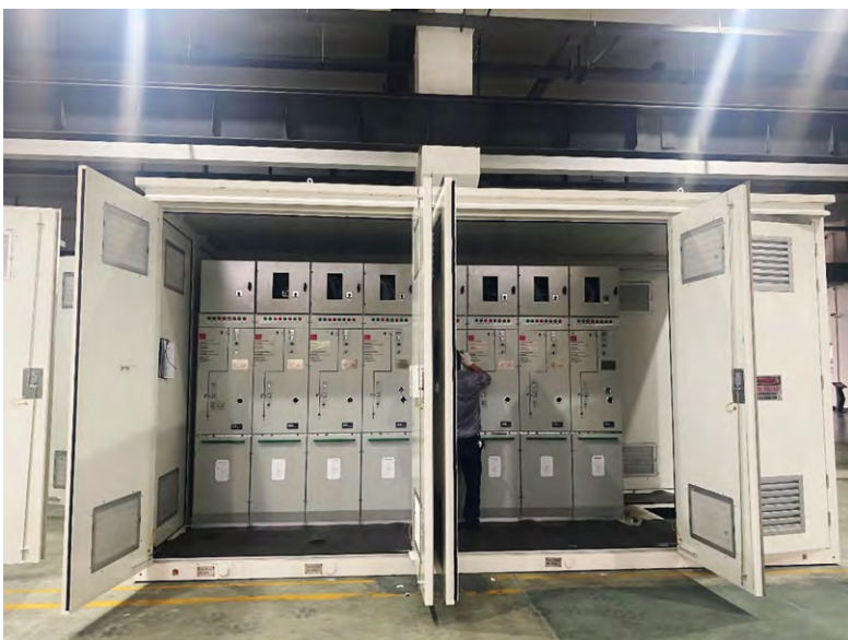
Secondary collector station
