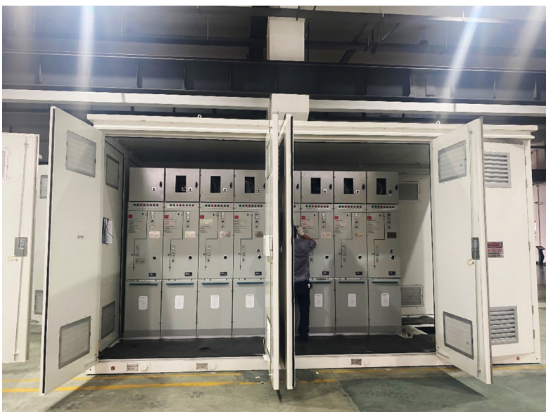
Secondary collector station (MV substation kiosk)
