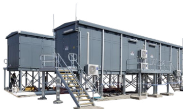
BGP-40.5 in a MV substation
