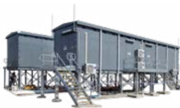
BGS-24 in a MV substation
