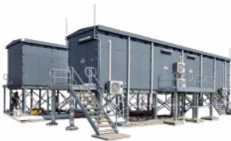
BGS-40.5 in a MV substation
